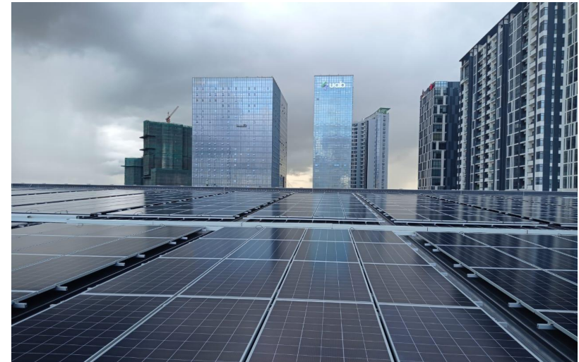
Commercial Rooftop Solar
