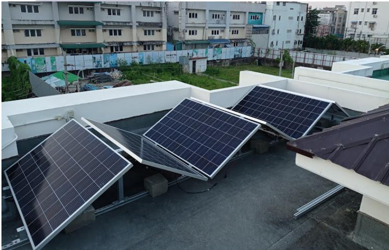
Residential Rooftop Solar
