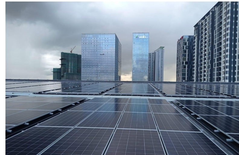
Commercial Rooftop Solar
